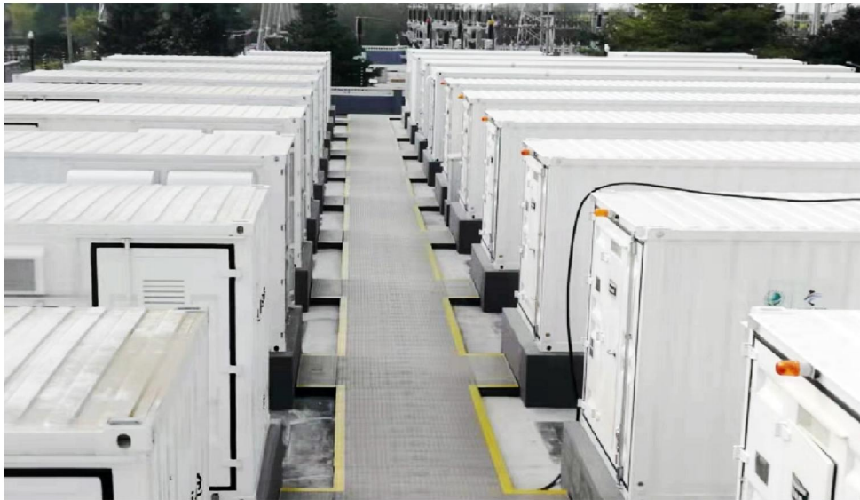
Box energy storage system in Henan longshan substation for peak load shifting
