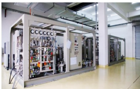
Central gas supply stations
