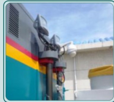
Lifting light and video monitoring system
