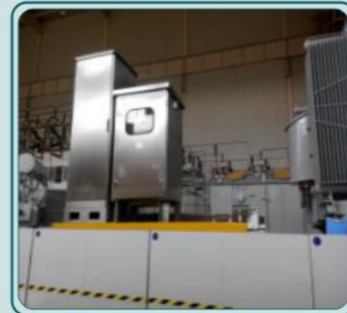
Transformer oil chromatography and terminal box
