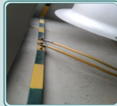
Grounding copper bar
