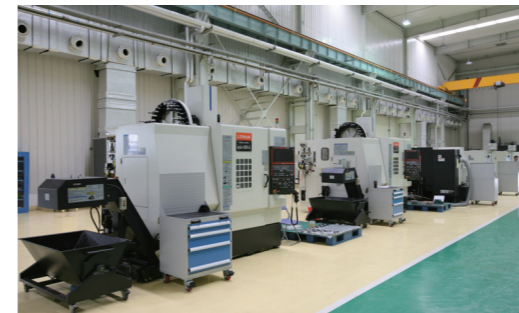
Digital processing and production line
