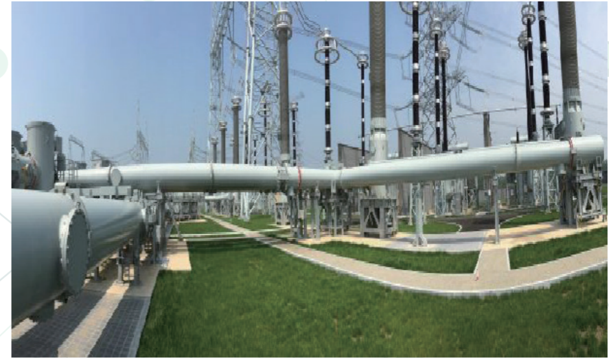
Import and export line of transformer substation
