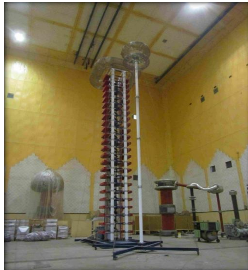
4800kV/480kJ impulse voltage generator
