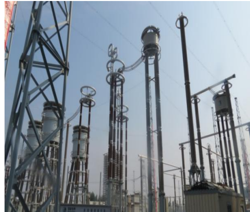
Zhongzhou converter station
