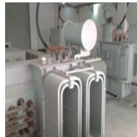
2500kVA temperature rise test system
