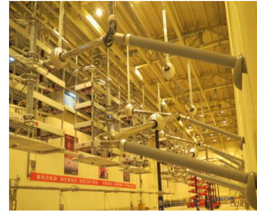
Jinhua converter station
