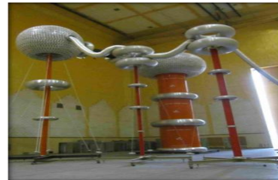
1800kV/7200kVA power frequency test system
